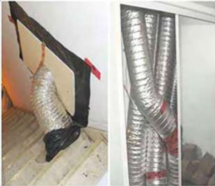
FIGURE 2. DO-IT-YOURSELF VENTILATION IN A COLORADO GROW HOUSE
